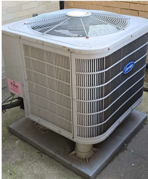
Photograph of the Equipment to be Replaced
